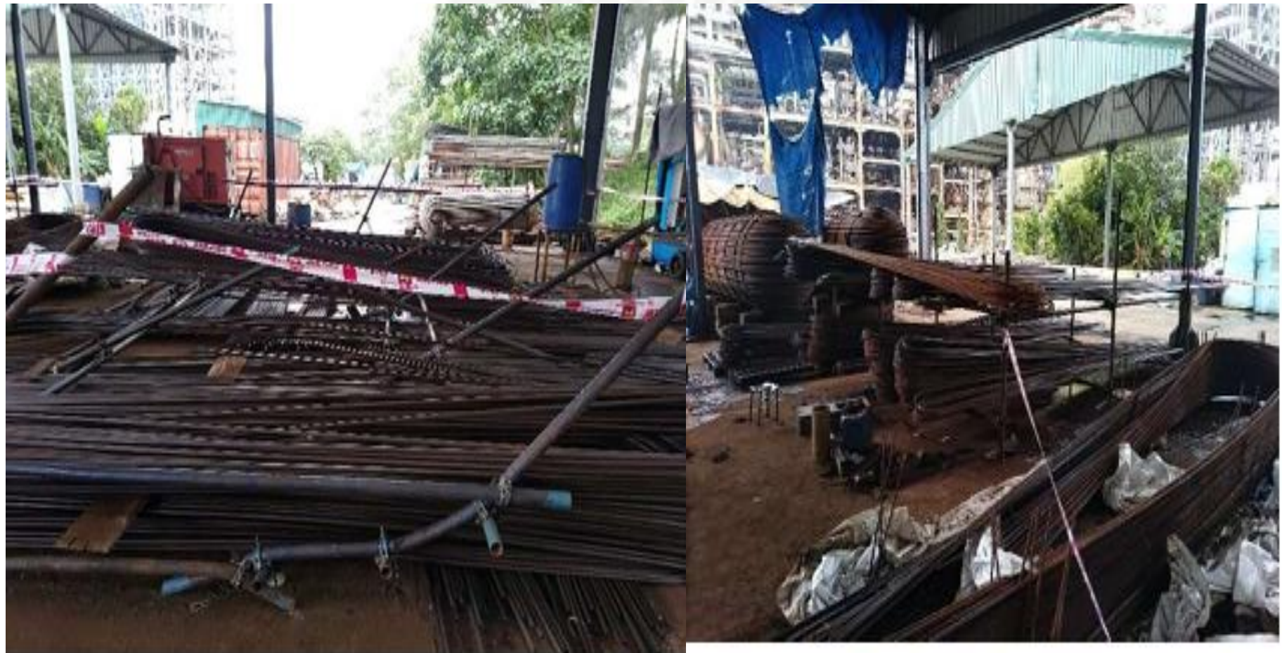
Collapsed structure without base plate, braces, safety signage
