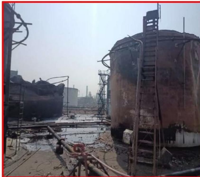
Figure 4: Image of the second exploded tank.
