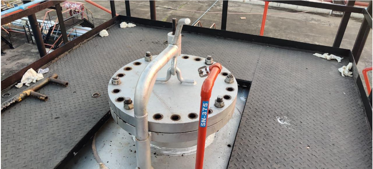
MANHOLE OF BULLET (460 MM INTERNAL DIA)
