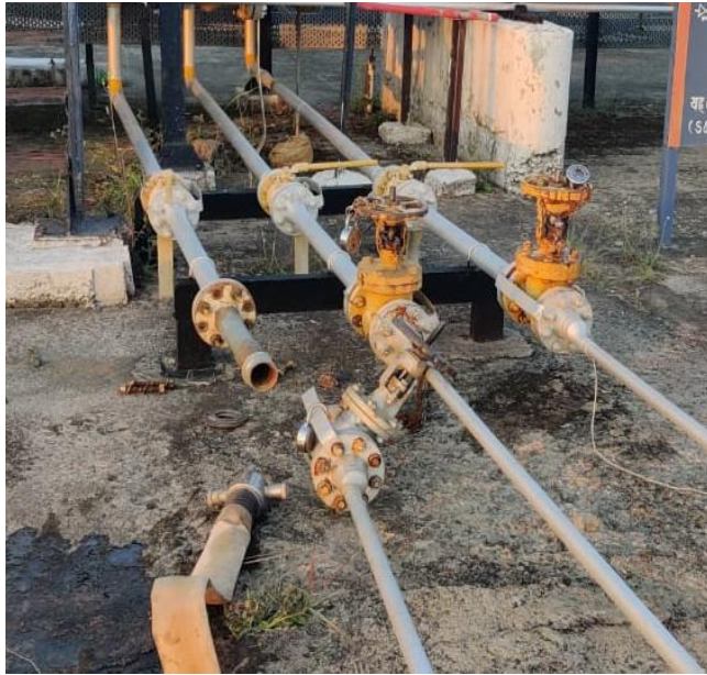
HOSE CONNECTION FOR WATER FILLING IN BULLET THROUGH WATER DRAIN LINE
