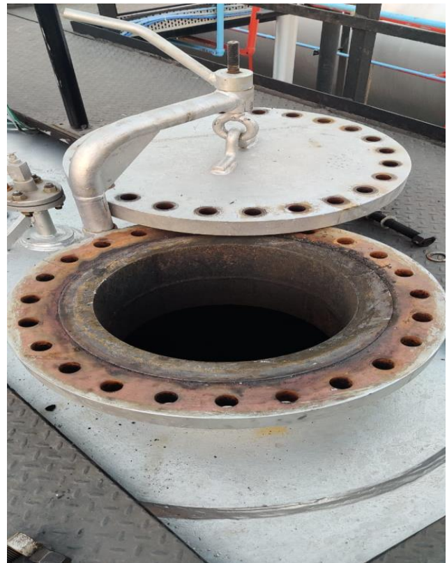
MANHOLE OF BULLET (460 MM INTERNAL DIA)
