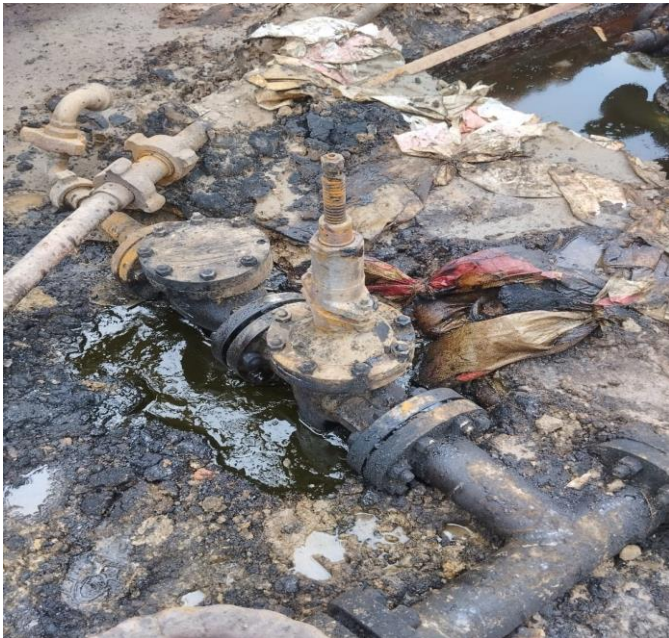
Flange between NRV & Gate valve that leaked
