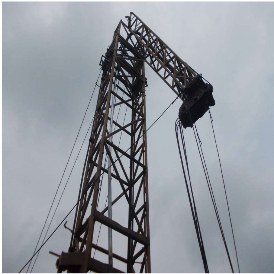
Photograph of broken telescopic mast
