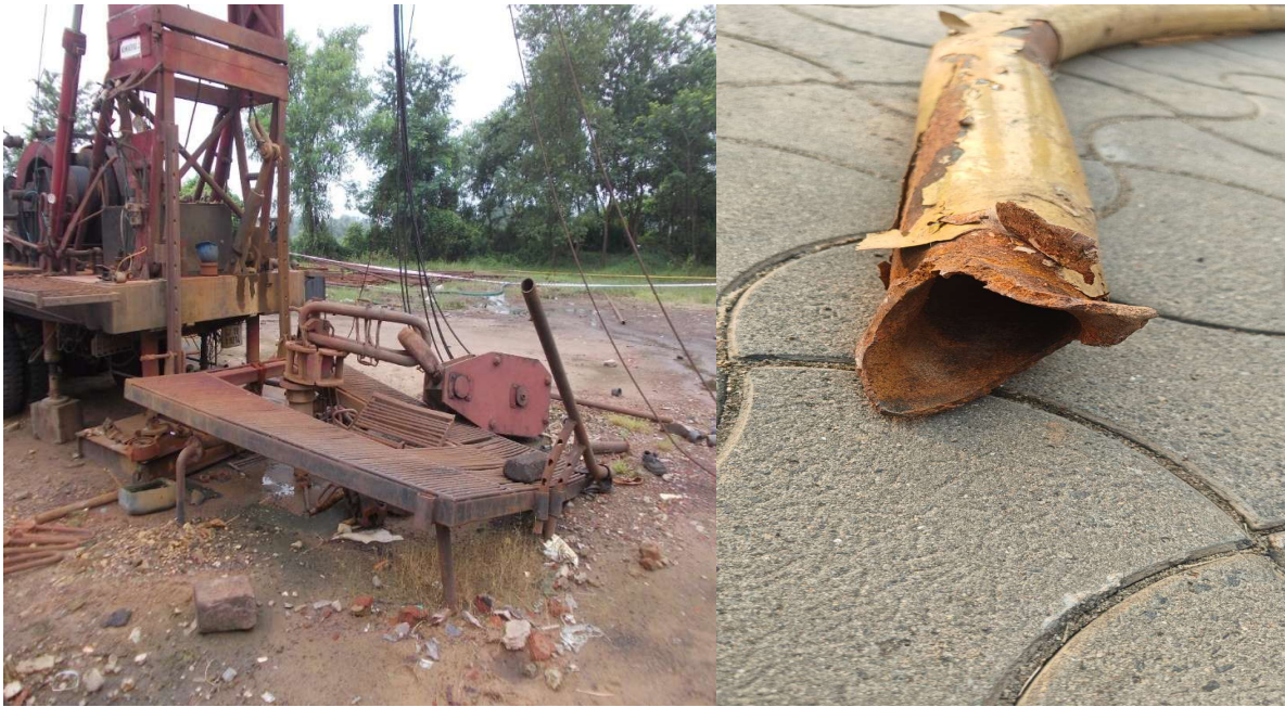
Photograph of fallen travelling block & broken metallic piece of Rig mast
