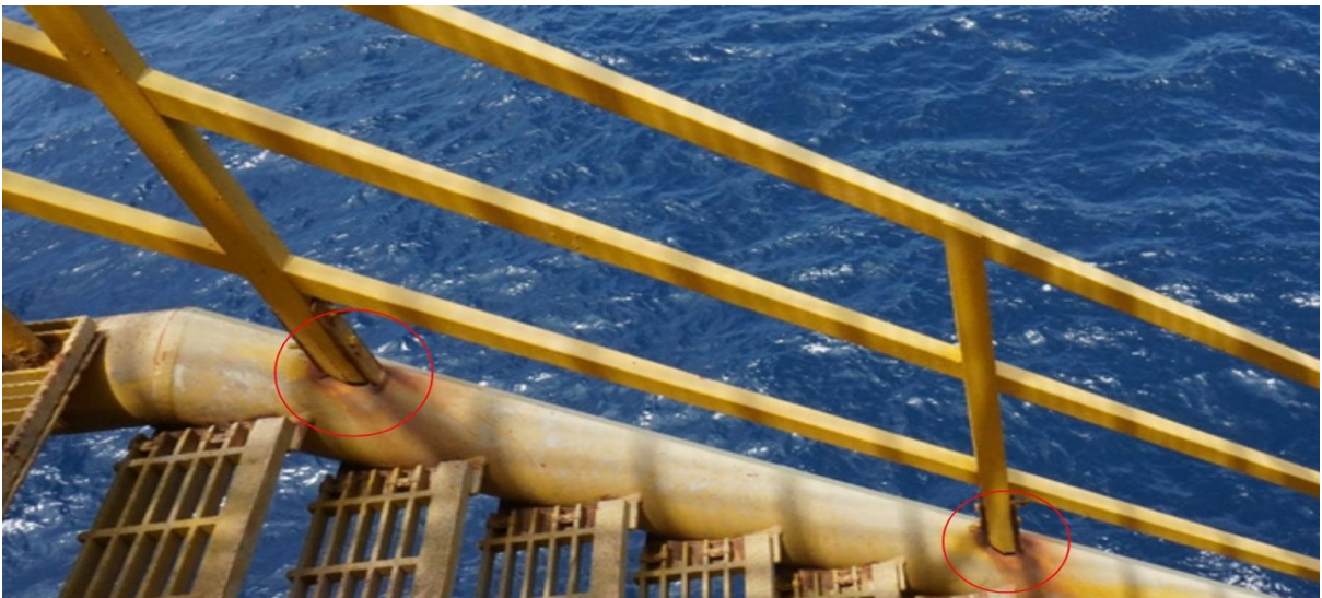
Photograph of cracks developed at the base of railing
