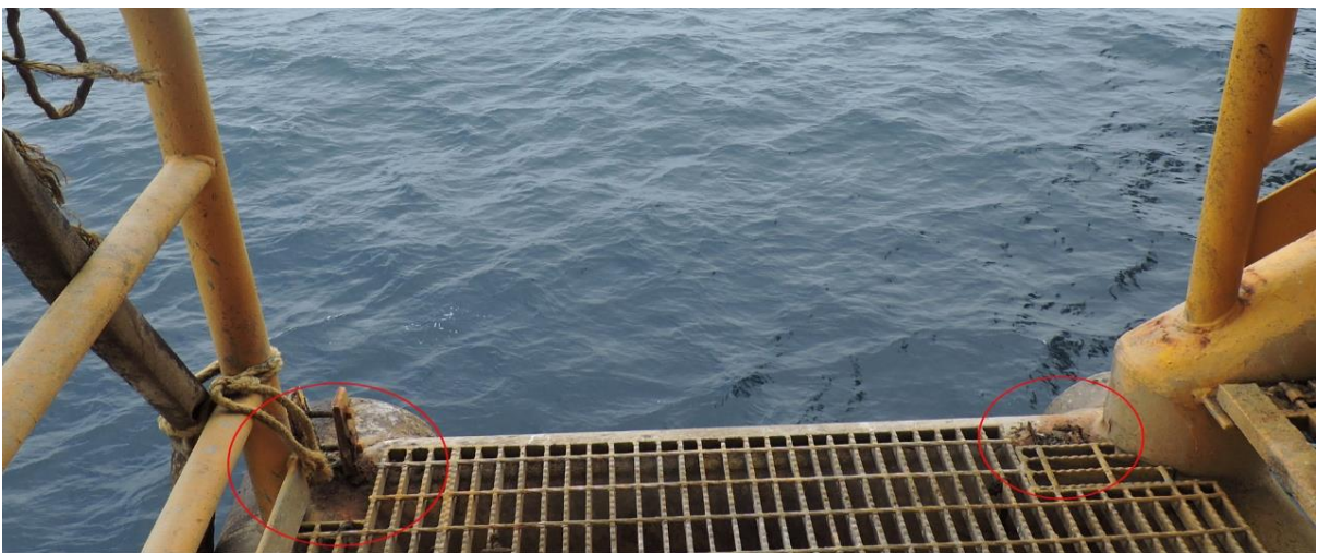
Photograph of broken railing
