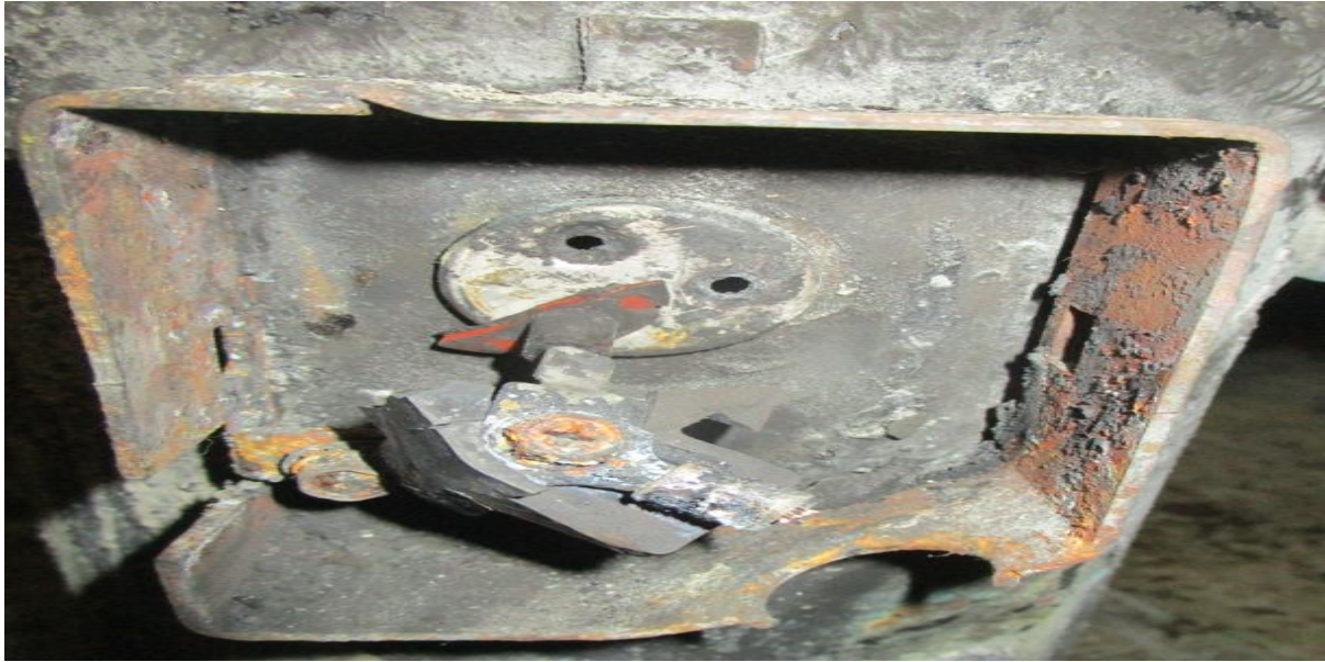
Figure 1: Terminal of the HVAC compressor after the incident
