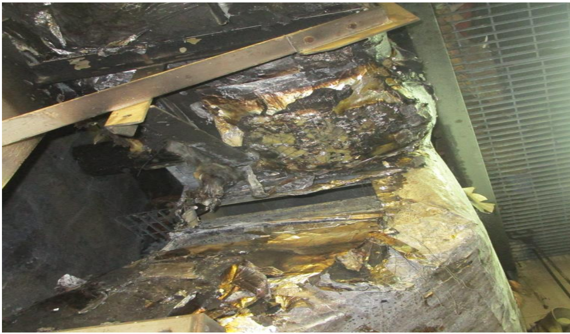
Figure 2: Damage to duct insulation of HVAC
